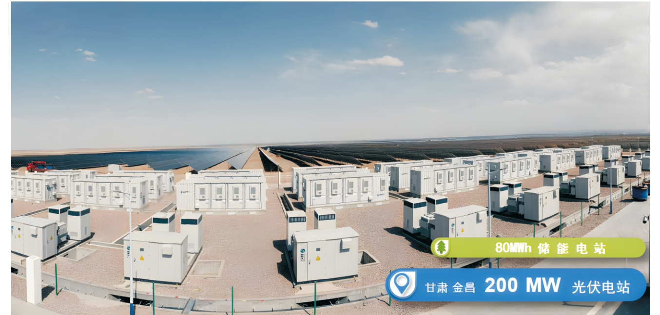
金昌—光储一体化项目 Jinchang - PV Power and Energy Storage Integration Project
